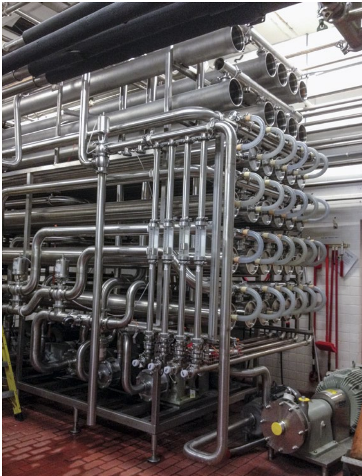
Figure 2 | Installation de filtration membranaire.
